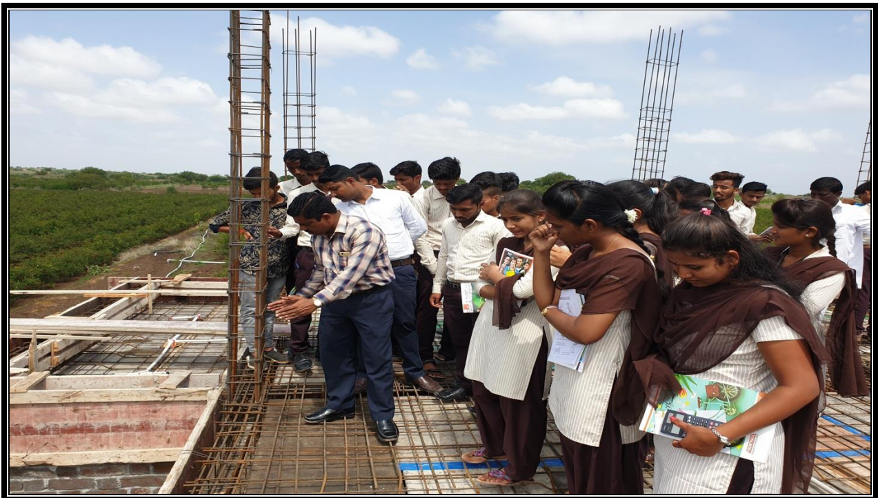
MR. DIGHE S.S EXPLAINING REINFORCEMENT DETAILS OF SLAB AT JAWALA ROAD KADLAS.
