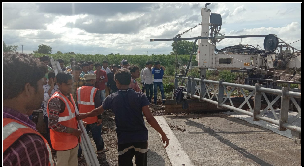
SITE ENGINEER HAS EXPLAINING DETAILS OF CONSTRUCTION OF CEMENT CONCRETE ROAD AT SANGOLA JATH ROAD [SH 71]
