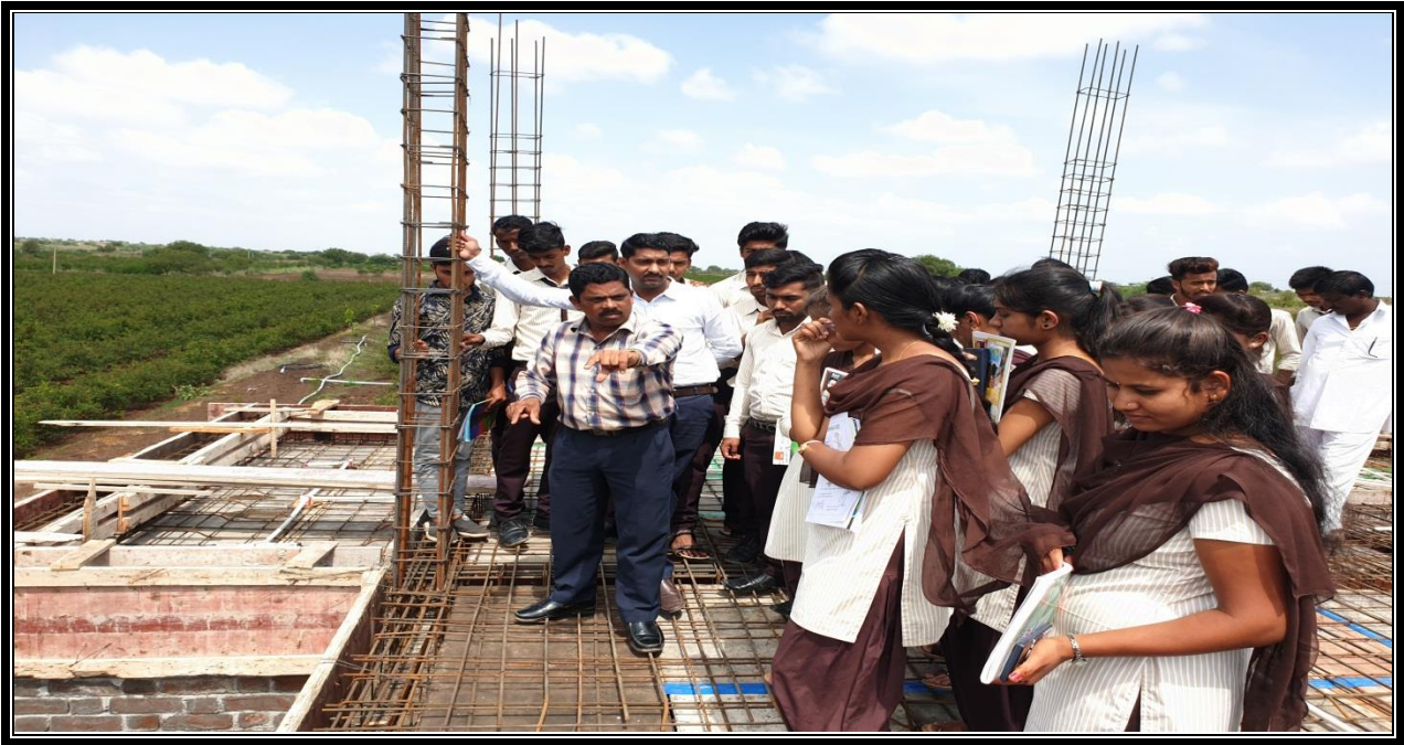
MR. DIGHE S.S EXPLAINING REINFORCEMENT DETAILS OF SLAB AT JAWALA ROAD KADLAS.
