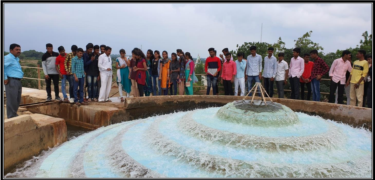
MR. MANE SIR EXPLAINING PROCEDURE OF WATER TREATMENT PLANT AT SHIRBHAVI, SANGOLA.
