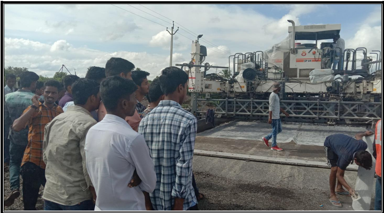
SITE ENGINEER HAS EXPLAINING DETAILS OF CONSTRUCTION OF CEMENT CONCRETE ROAD AT SANGOLA JATH ROAD [SH 71]
